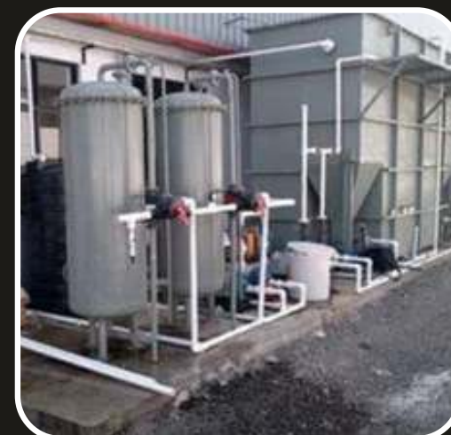
Grey water treatment
