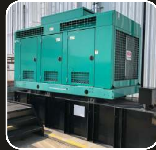
Generator backup for common areas
