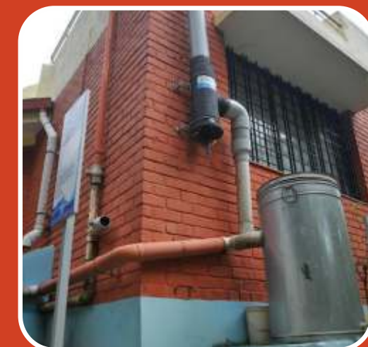
Rain Water Harvesting
